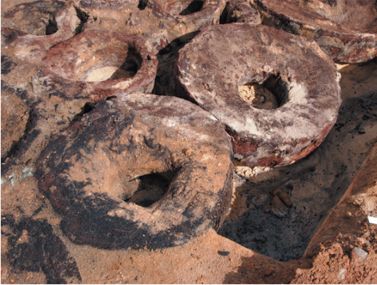
Some of the jarrah rounds known as 'Hampton's cheeses' being dug up from the highway. (Photo courtesy Bridget Curran.)
